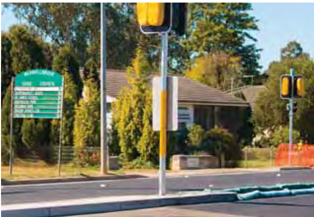
Traffic lights being installed at intersection of Rutherford Road and New England Highway in August this year.
